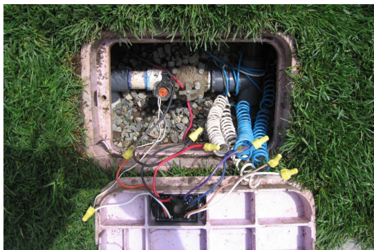
Pathway FM Module installed at “Host” Zone Valve
